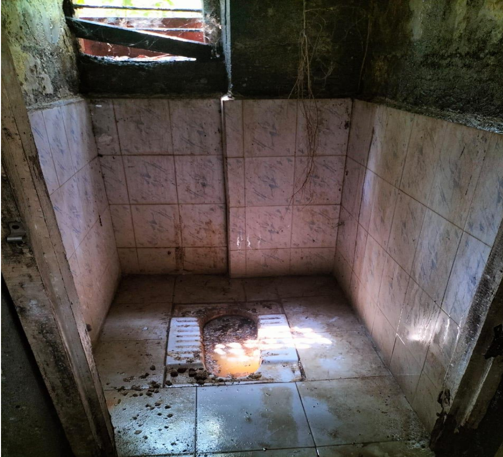
Choked Toilet in Female ward no. 18
