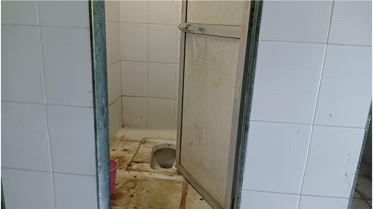
Fig:3 Pathetic Condition of the toilets on the academic floor
