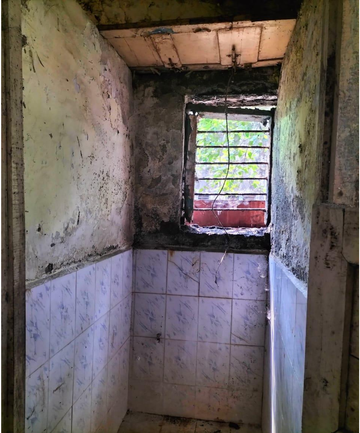
Broken window in Female ward number 18
